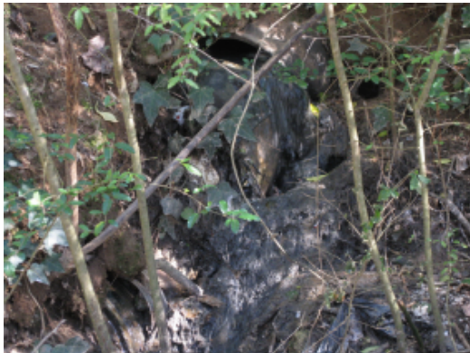
Broken sewer line on tributary of Long Island Creek
