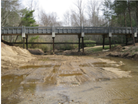
Evidence of vehicles driving through stream
