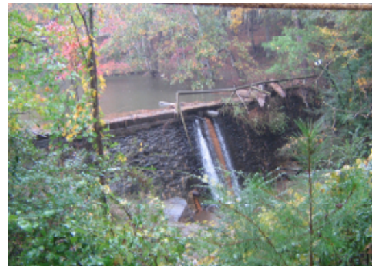
Water quality and channel protection benefits could be achieved by re-designing the outlet control structure at this existing pond as part of Project 06 0353 LL012-BMP-1
