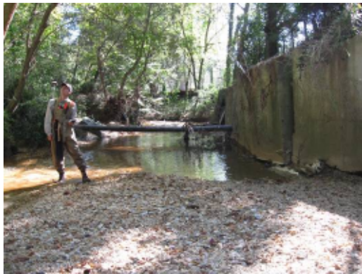
Channelized reaches were observed in densely developed areas such as this stream crossing with Roswell Road
