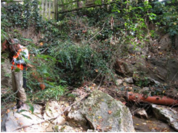
Bank failure exposed and cracked clay sewer line
