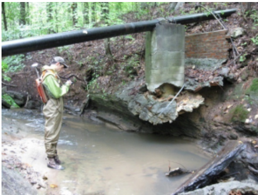
Undermined sewer crossing support
