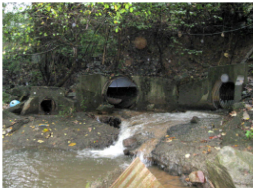
Several outfalls draining commercial and high density residential land near Northridge Crossing Drive
