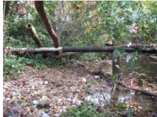
Exposed PVC sewer pipe with debris loading
