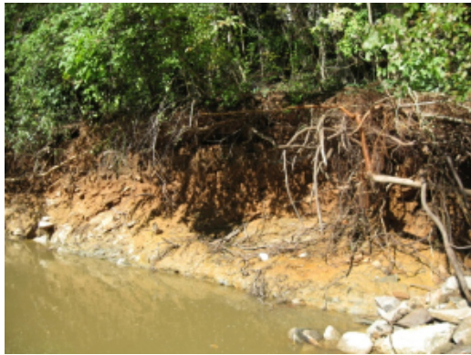
Example of bank erosion in the 75-100% range
