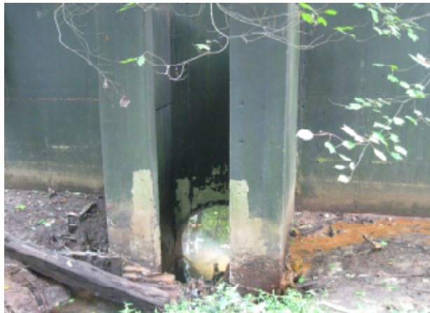
Modification of this outlet structure would increase water quality benefits as part of project 17 0024 LL084-BMP-1
