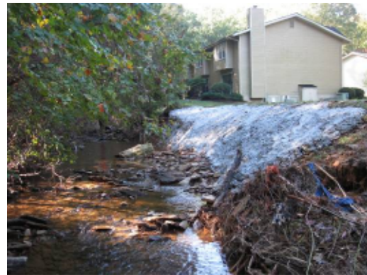
Riprap lined banks were the most commonly observed man-made alteration
