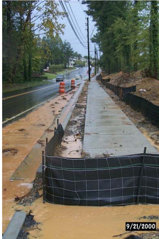
FIGURE 3-1 Direct Runoff of Sediments at Construction Site
