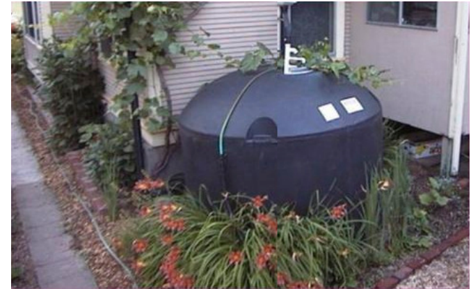
Figure 1 | 1500 gallon cistern (LID Urban Design Tools via City of Atlanta)
