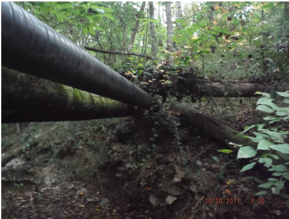
Figure 3-7 Fallen tree along tributary to Nancy Creek in Subwatershed NC08 (MP#1035)
