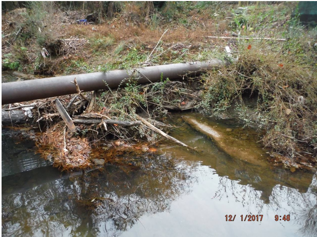
Figure 3-29 Debris Dam on Sewer Crossing in Subwatershed LI04 (MP#1093)
