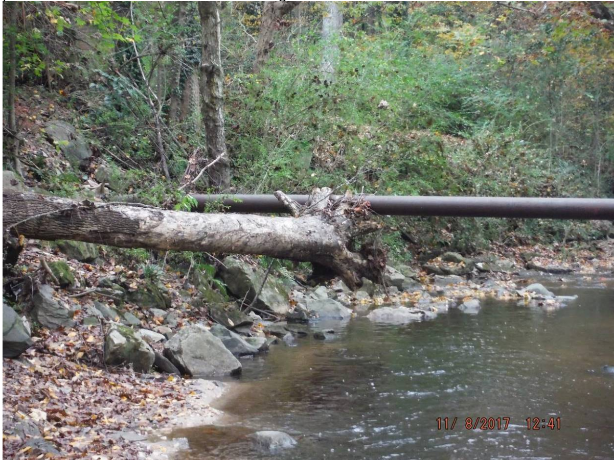
Figure 3-19 Sewer Crossing in Subwatershed MC04 (MP#1050)
