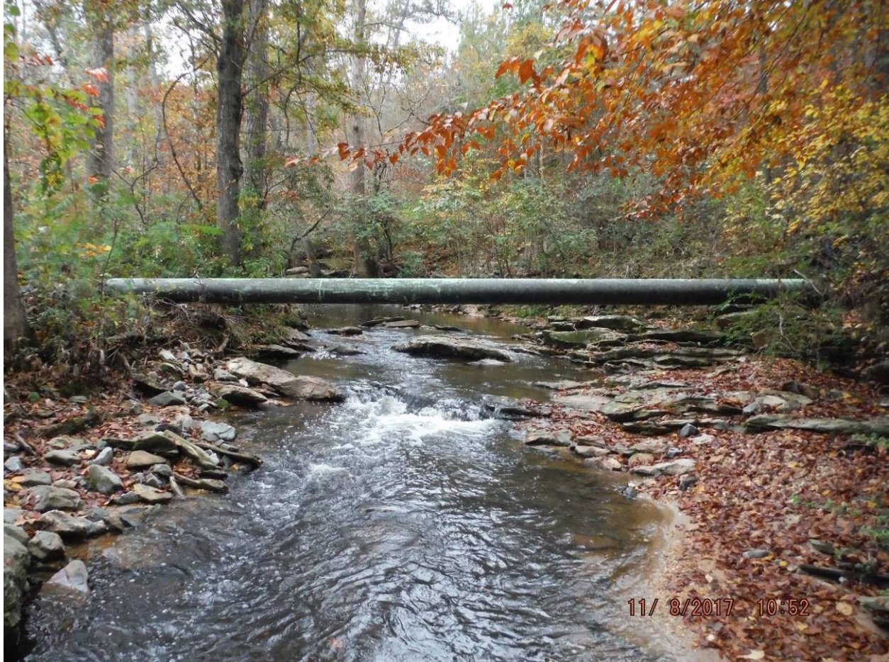
Figure 3-18 Sewer Crossing in Subwatershed MC03 (MP#1049)
