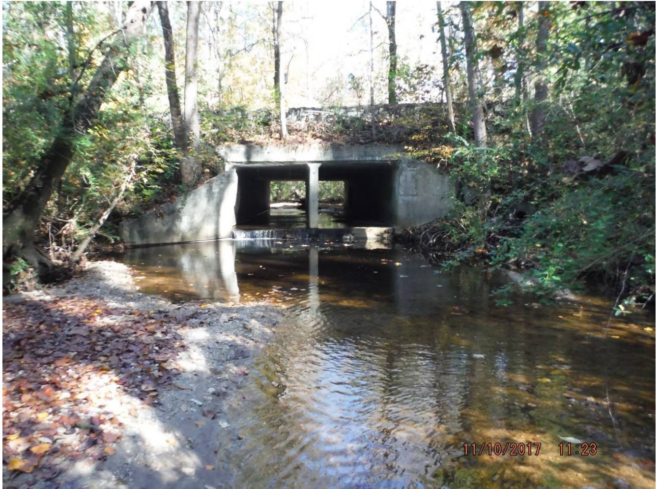
Figure 3-21 Glenridge Parkway Culvert and broken headwall in Subwatershed MC06 (MP#1061)
