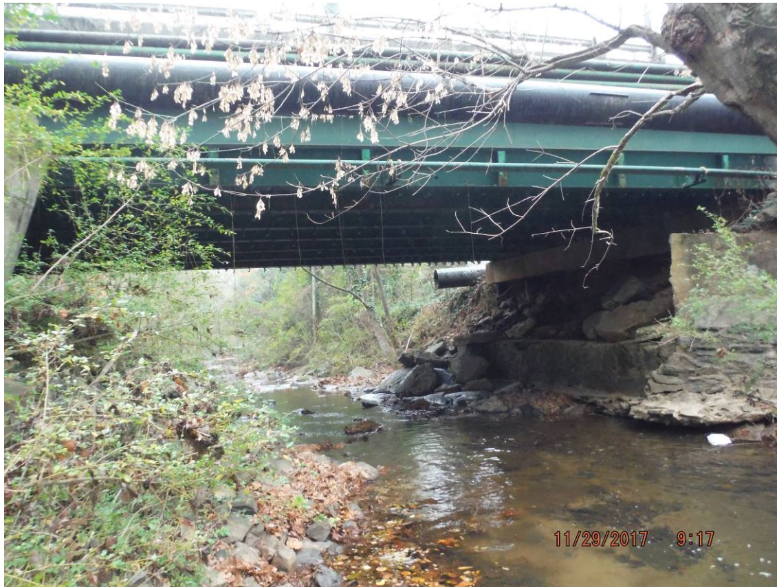
Figure 3-27 Structural damage to bridge footings in Subwatershed LI02 (MP#1092)
