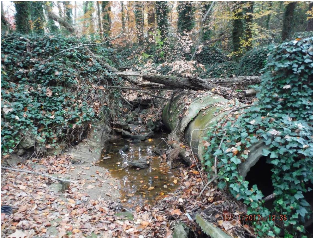
Figure 3-31 Concrete Pipe Debris in Subwatershed LI06 (MP#1098)
