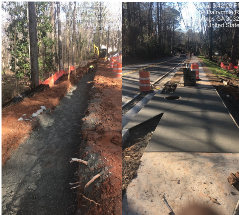
TS168 Dalrymple Sidewalk Retaining Wall Foundation and Sidewalk Storm System and Sidewalk Installation
