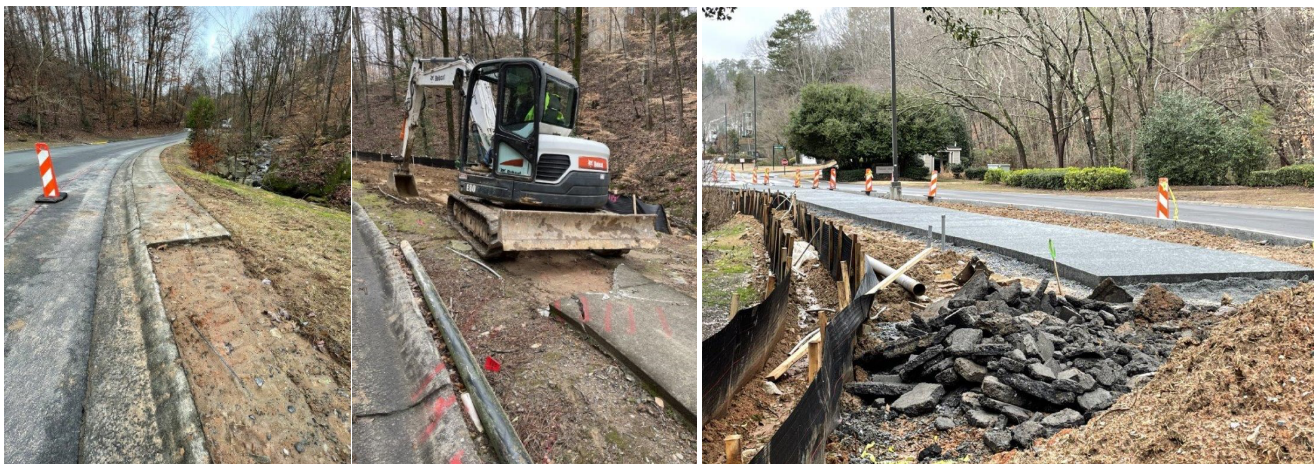
Trail 2A (left to right): End of Demolition, Demolition Resumes, Pervious Surface
