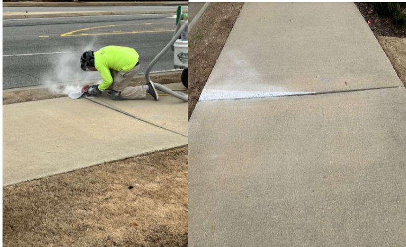
Sidewalk trip hazard repairs
