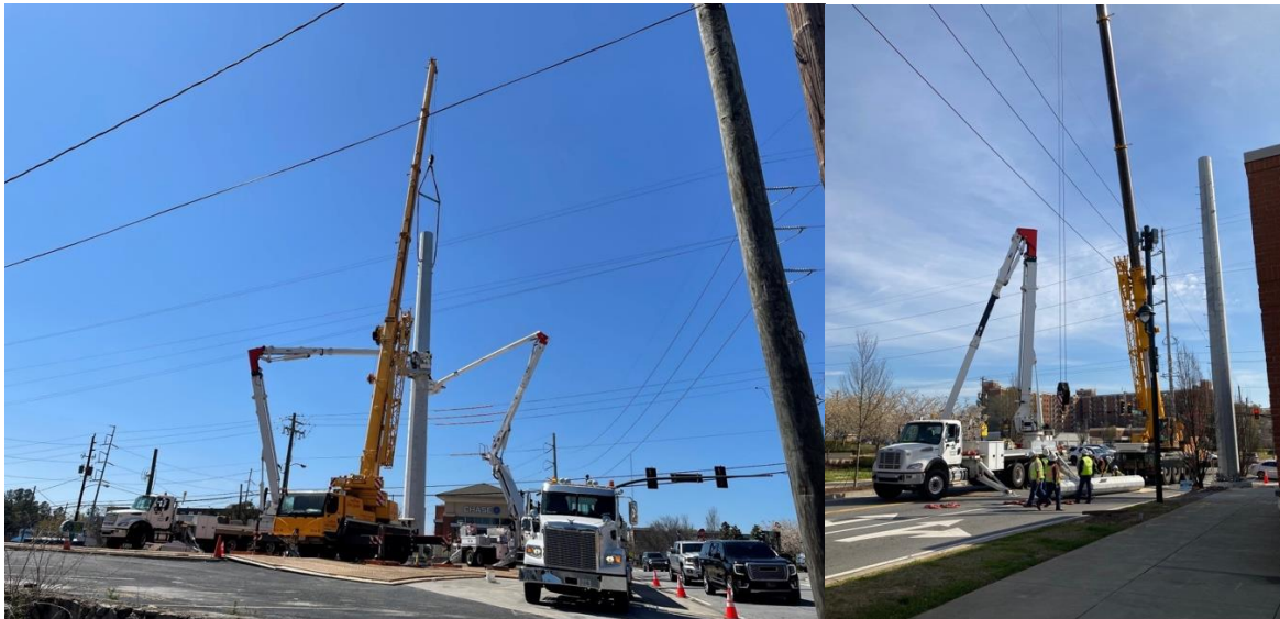
TS-191 Mt. Vernon at Roswell Road Georgia Power Company transmission tower installation
