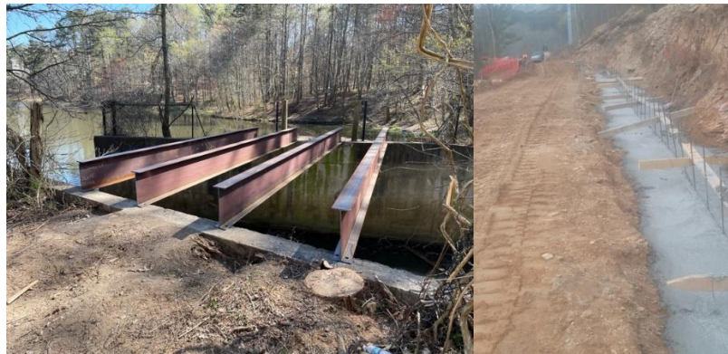
Trail 2A (left) Spillway Bridge was Demolished and Steel Beams Placed for Replacement, (right) North Side of Orkin Lake, 225' of Concrete was Poured for Wall Footers
