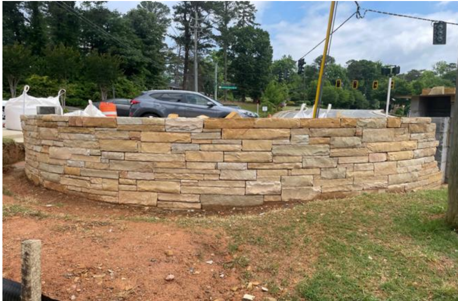
Stone Cladding Installed on Pedestrian Landing Walls at Johnson Ferry Road and Abernathy Road
