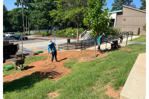
Hammond Park Erosion correction.
