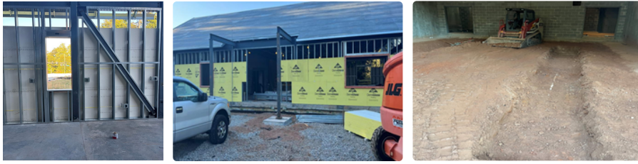
Photo Description (left to right): Continue MEP Inwall Rough In and Sheathing, Sheathing Installation on Both First and Second Floor, Prepping Apparatus Bay for Slab on Grade Pour
