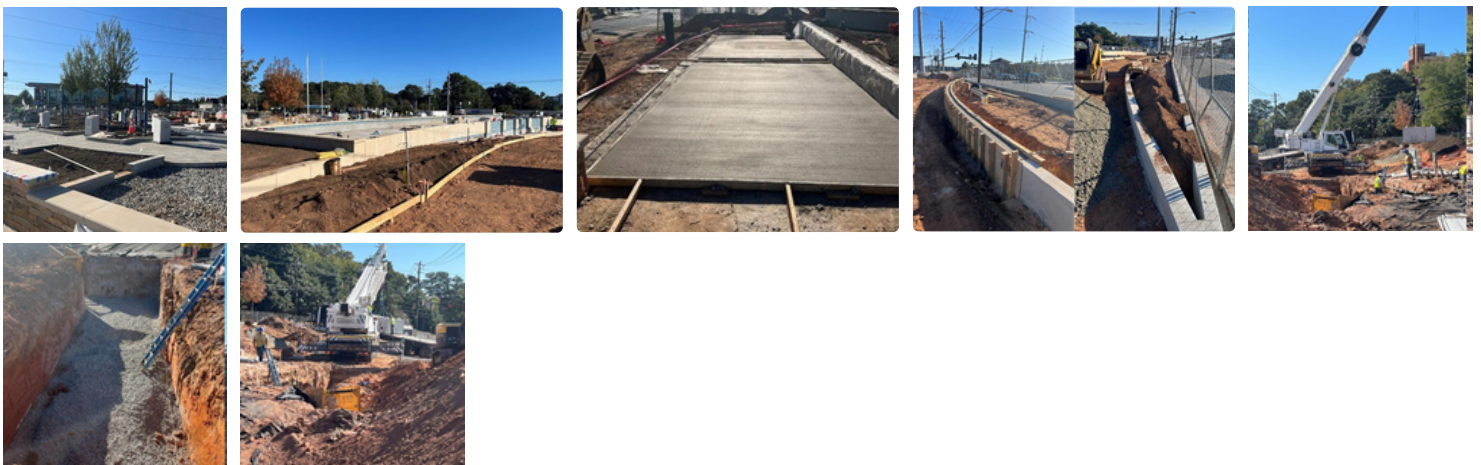
Photo Description: Top (left to right) - Install of bluestone pavers & monuments, Fountain Finishes - Tile and Veneer, Mt. Vernon Sidewalk final section, Seat Wall & Planter along Roswell Rd, Prep for sidewalk along Roswell Rd, GA Power prep and set electrical vaults. Bottom (left to right) - GA Power prep and set electrical vaults
