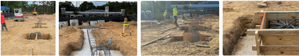
Photo Description (left to right): Begin Pouring Footings and Piers, Finishing Pouring Building Footers, Prep for pouring piers, Prep for pouring piers
