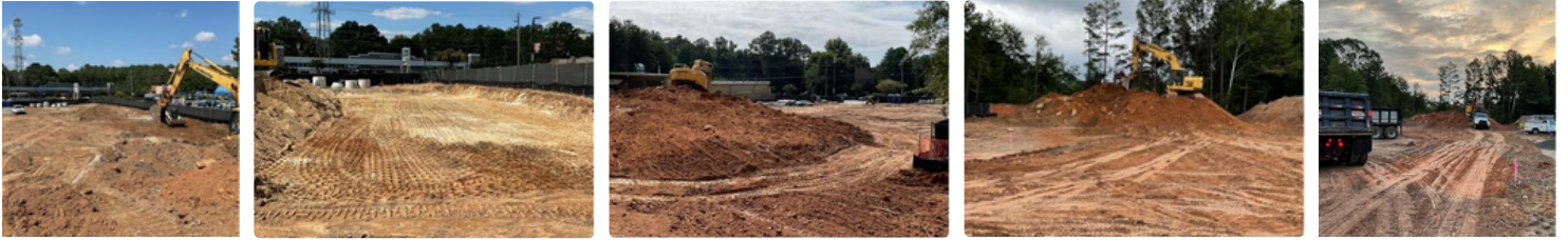
Photo Description (left to right): Continued Building Pad Preparations, Continued Building Pad Preparations, Continued Grading, Continued Grading, Continued Export of Dirt and Unsuitable Materials
