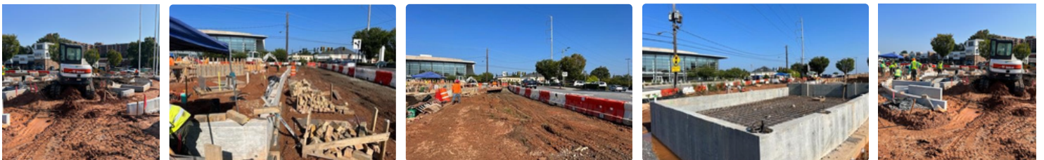
Photo Description (left to right): Prepping soil inside granite slabs & prepping pedestrian area for sub-slab pour, Work on upper Johnson Ferry Wall veneer, Commenced work along Johnson Ferry Road, Lower basin slab ready for pour, Prepping soil inside granite slabs & prepping pedestrian area for sub-slab pour
