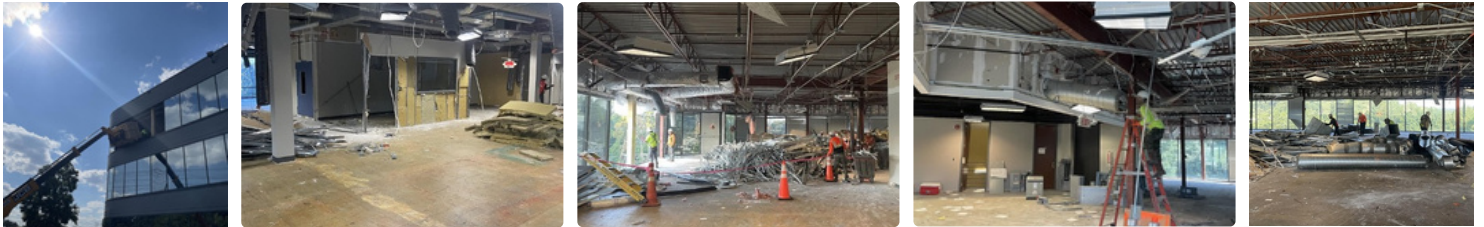
Photo Description (left to right): Exporting Demolished Materials, Demolishing Existing Conditions, Demolishing Existing Conditions, Connecting Temporary Light and Power, Demolishing Existing Conditions
