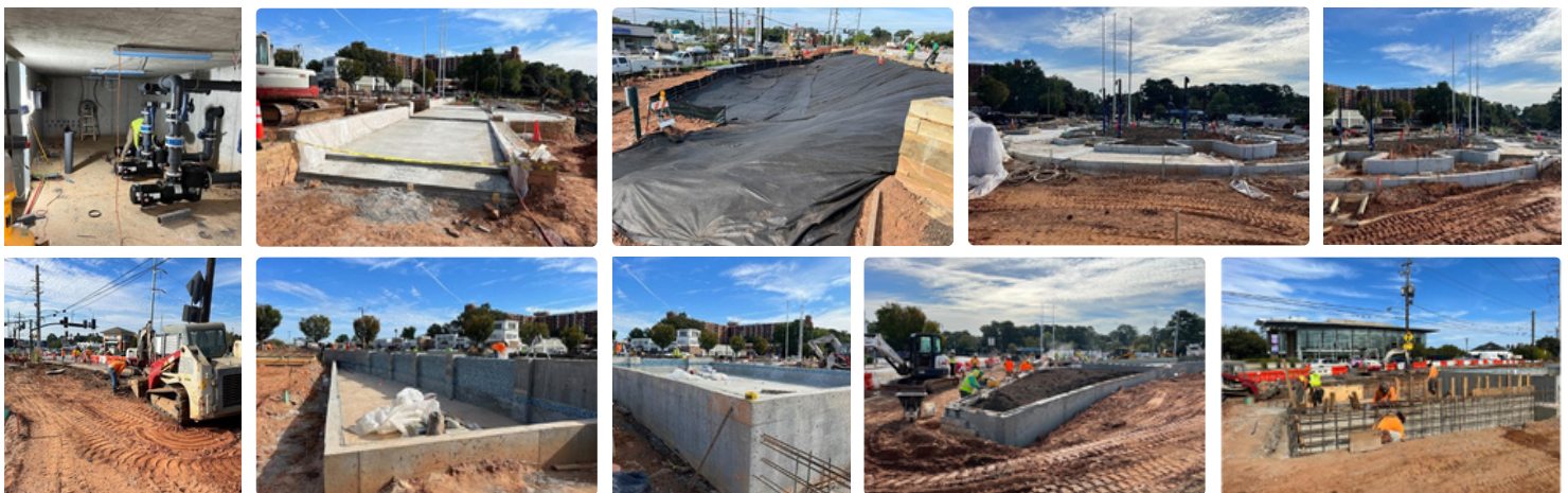
Photo Description: Top (left to right) - Began install of equipment in vault, Completed pour of middle and eastern section of Mt. Vernon sidewalk, Began demo of sidewalk along Roswell Road, Installed site lighting in monument area. Bottom (left to right) - Installed site lighting in monument area, Continued install of tile in fountain basins, prepping Roswell Road planters.
