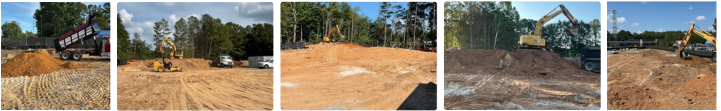
Photo Description (left to right): Hauling In Material to Begin Backfilling the Building Pad, Continued Grading, Continued Export of Unsuitable Materials and Dirt, Continued Building Pad Preparations
