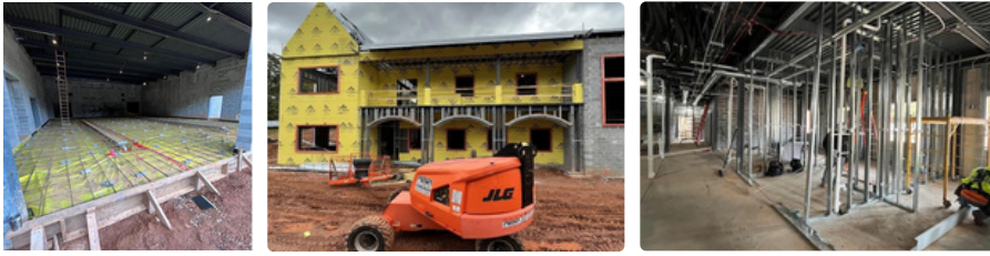
Photo Description (left to right): Completed Concrete Prep at Apparatus Bay, Completed Exterior Sheathing on First and Second Floor, Began Interior Framing on First Floor.
