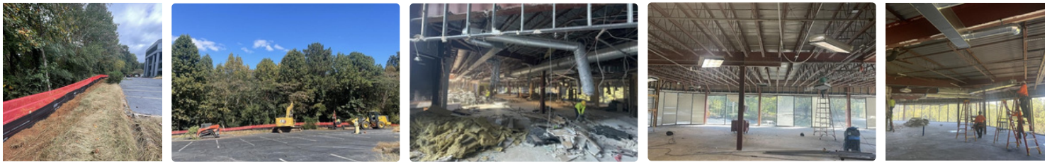
Photo Description (left to right): Clearing And Grubbing Of The Site, Clearing And Grubbing Of The Site, Demolition Of Interior Walls/Ceilings/Flooring, Complete Joist Augmentation On Level 3, Overhead MEP Rough-in On Level 3
