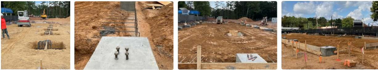
Photo Description (left to right): Pouring Footings and Piers, Finish Pouring Footings and Piers, Prep Slab For Concrete Pour
