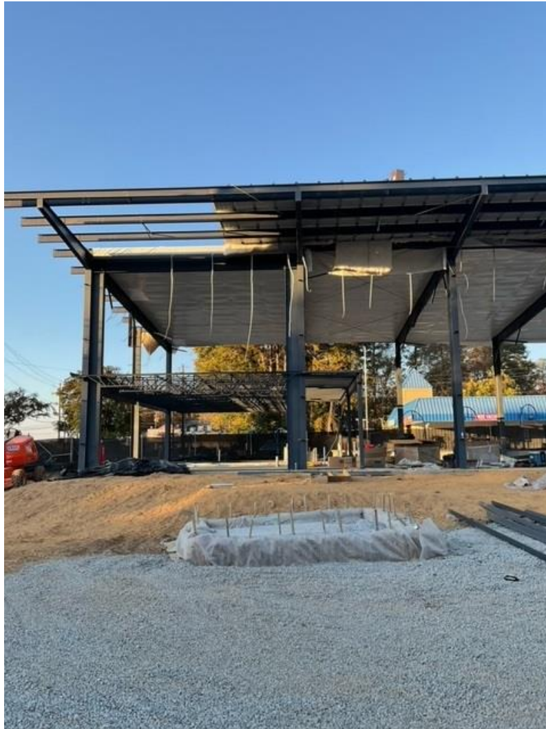
Installation of insulation on top of the fabric liner; Installation of decking of the mezzanine.
