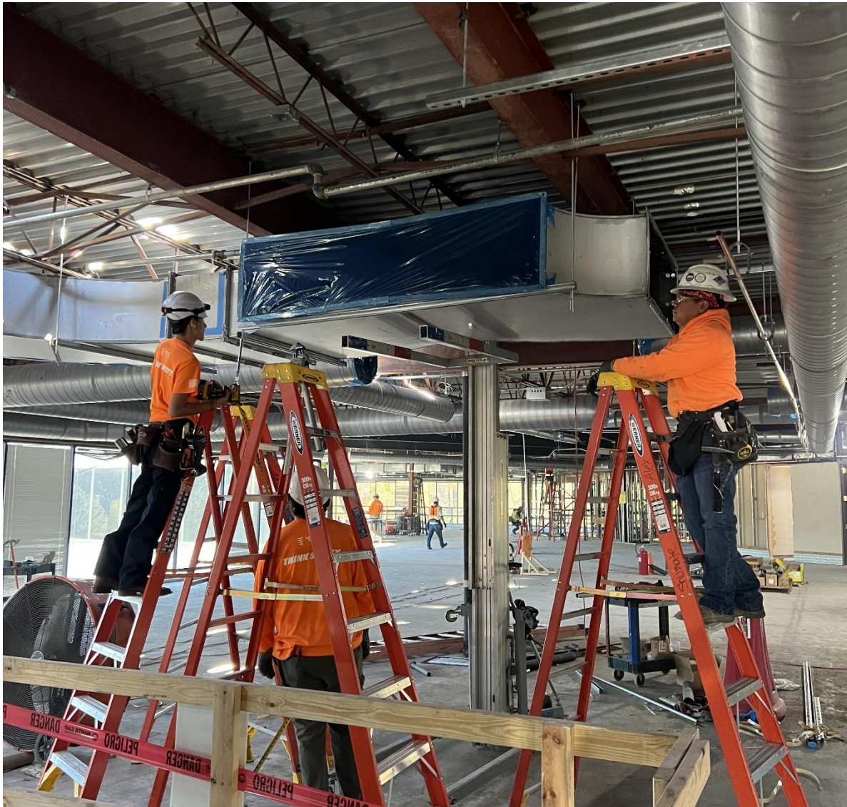
Mechanical Overhead Rough-In
