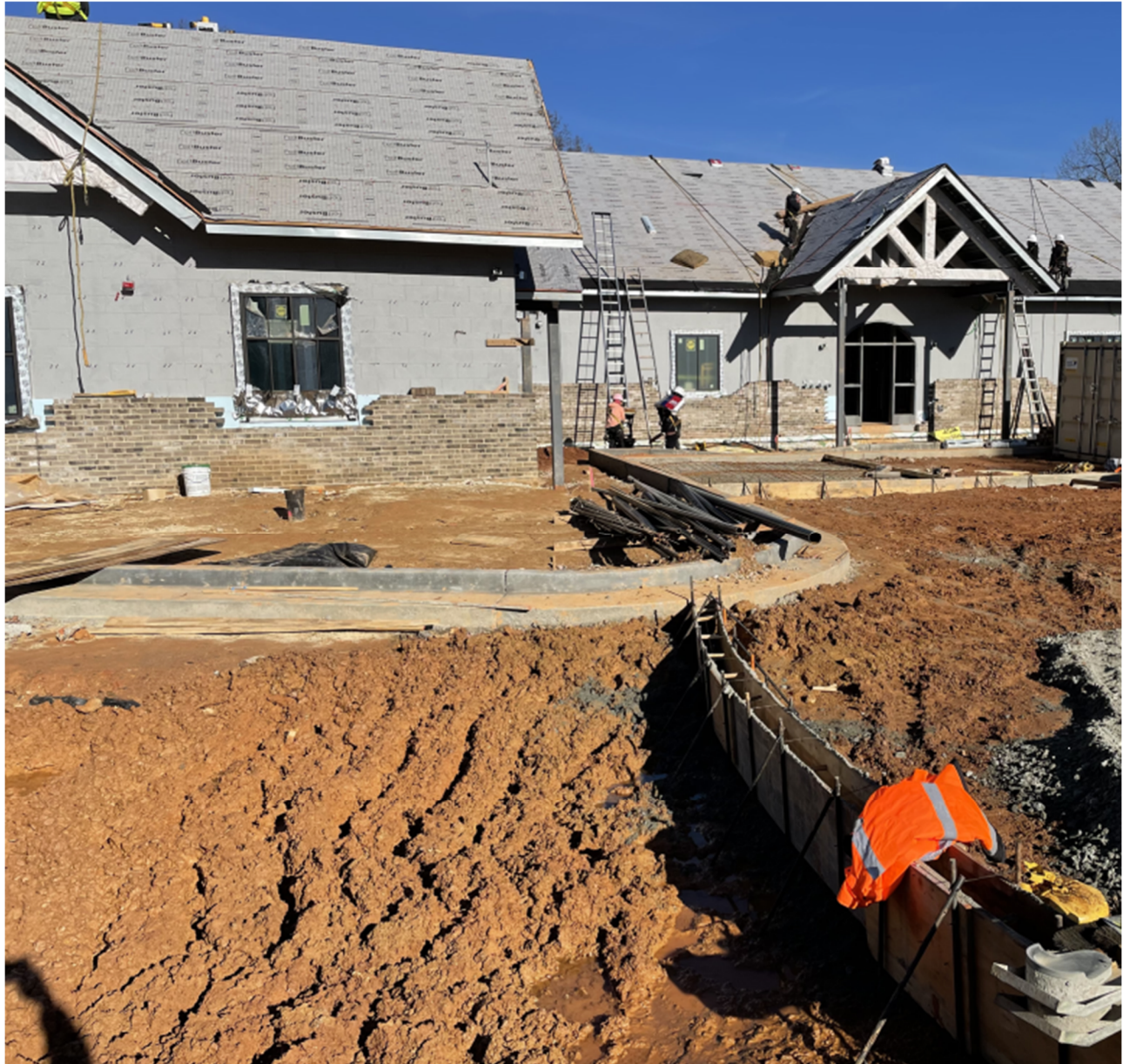
Began Installing Header Curb and Sleaving and Prep for Mt Vernon Parking Lot
