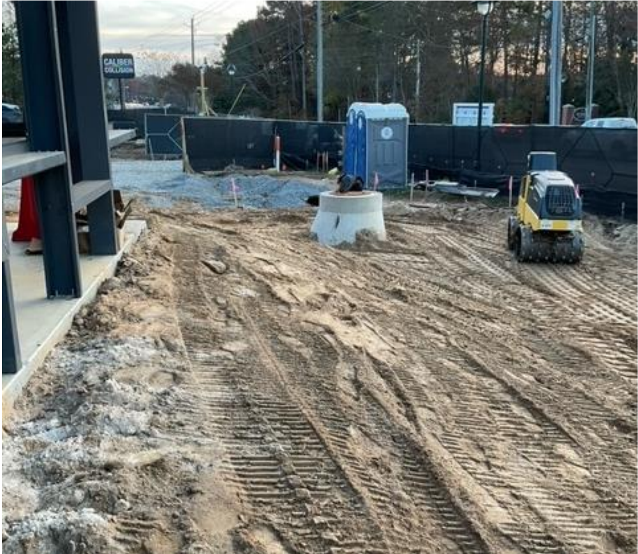
Installed Sanitary Sewer System
