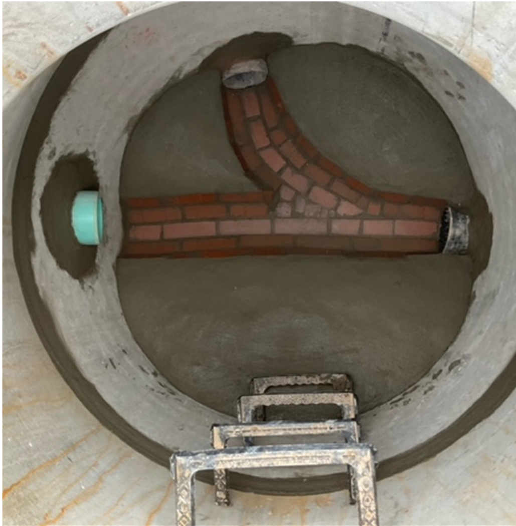
Installed Sanitary Sewer Inverts
