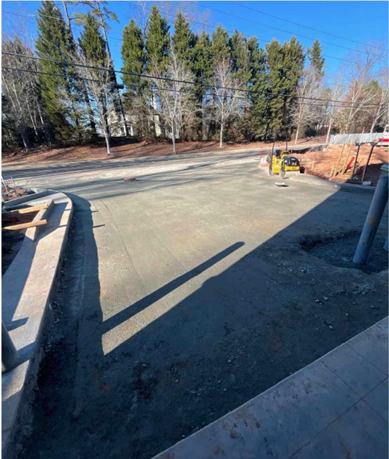
Began Prepping for Concrete Apron at Spalding Dr Entrance and Apparatus Bay
