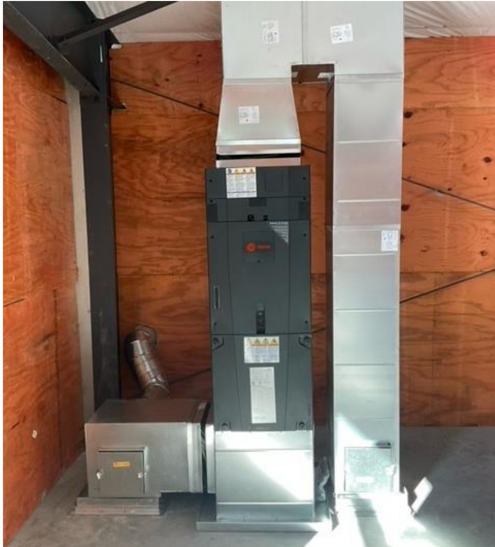
Air Handler Installed
