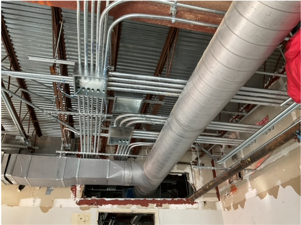
Mechanical O/H & In-Wall
