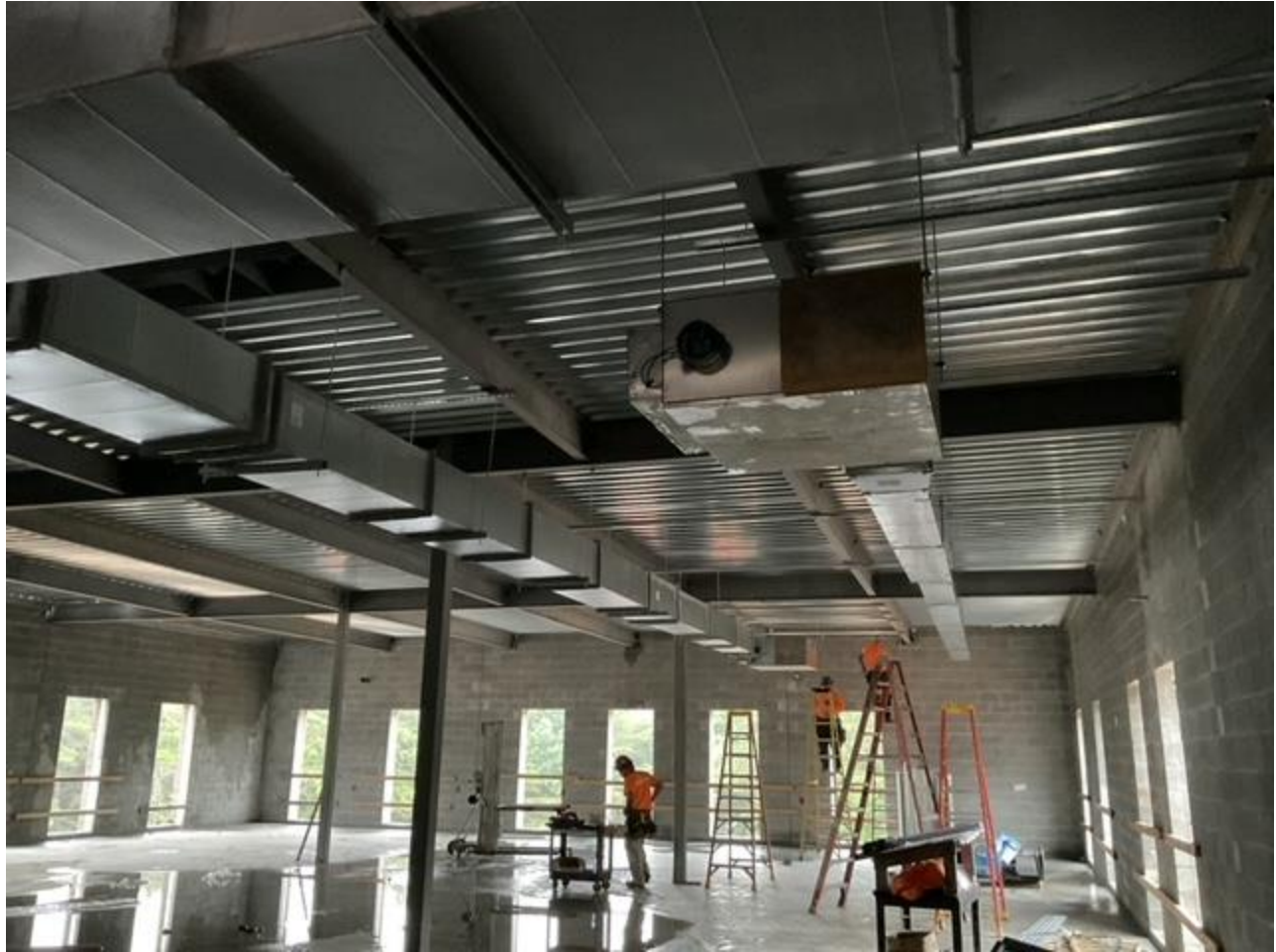
Overhead Mechanicals at Sally Port
