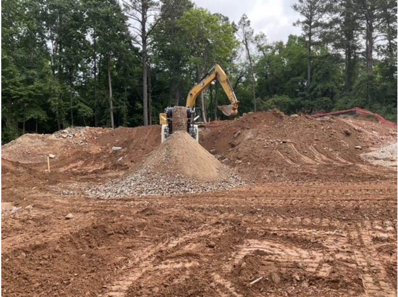
Rock Crusher Operations
