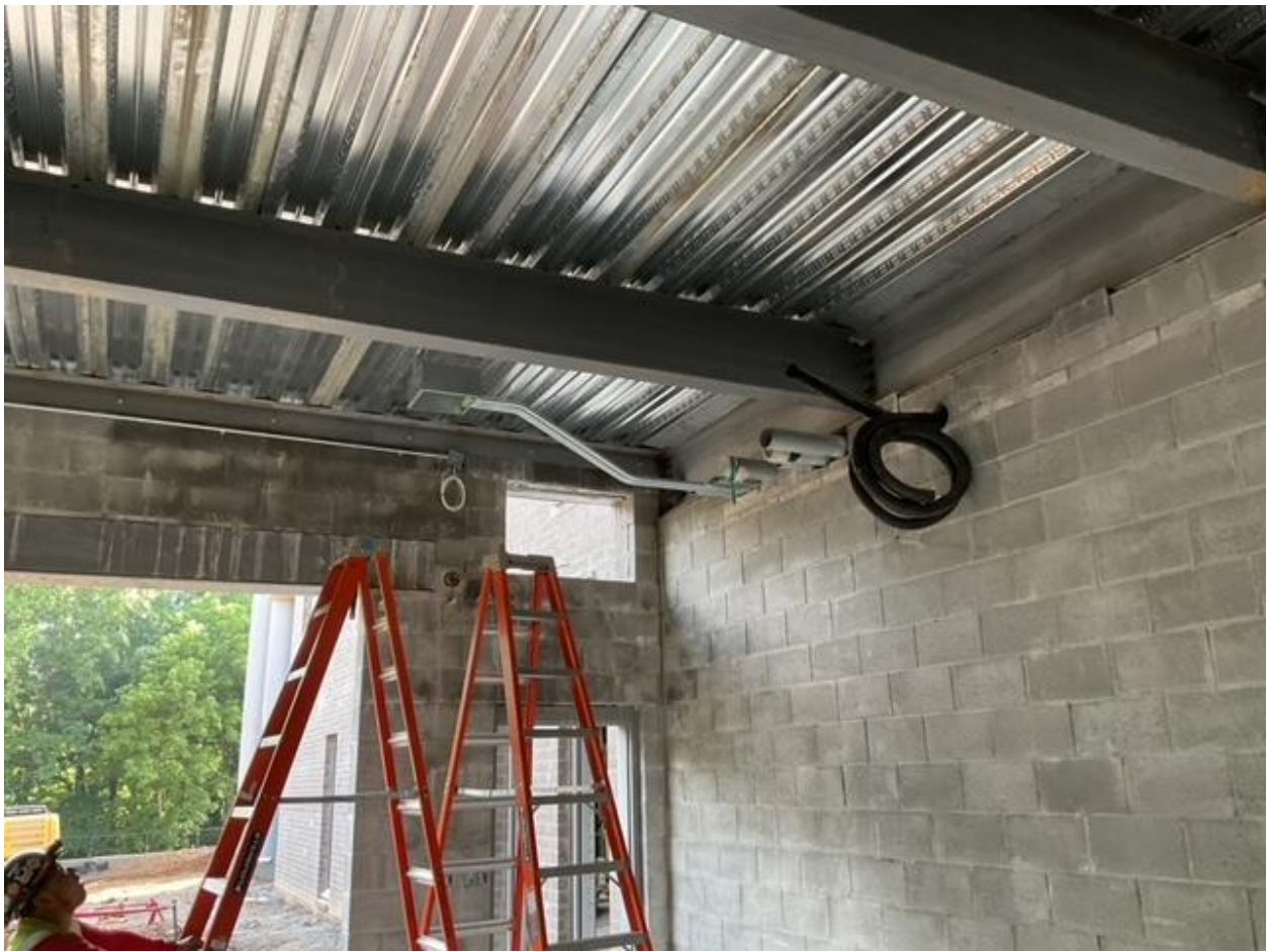
Electrical Overhead @ Sally Port
