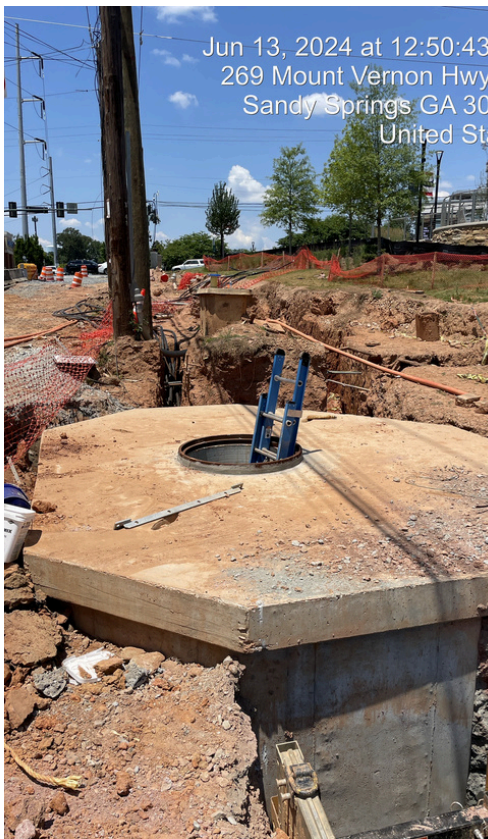
TS191 Utility Vault Supporting Aerial Utility Undergrounding at Veterans Park
