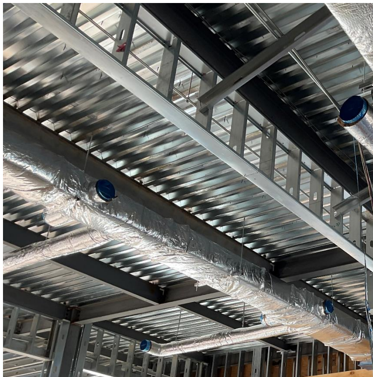
Overhead MEP at Courts Addition
