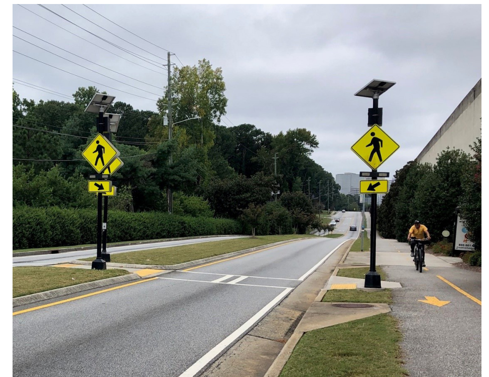
Rectangular Rapid Flashing Beacons (RRFB)
