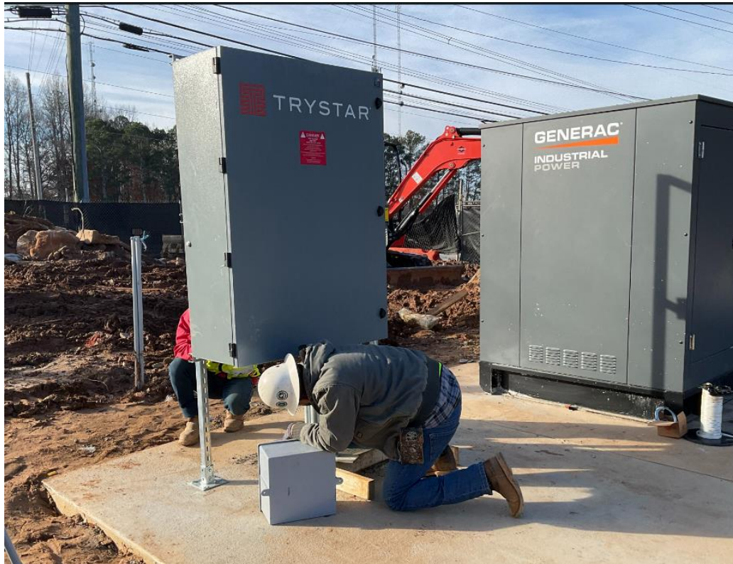
Automatic Transfer Switch for Generator
