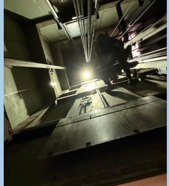
Sandy Springs Fire crews trained on elevator training and rappelling for the inevitable stuck elevator calls that occur within the several highrise buildings in the City.
